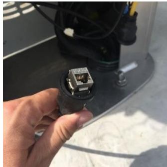
Figure 21: Terminated Ethernet jack.
