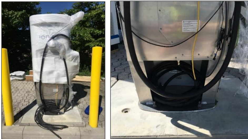
Figure 17: Mounted UU, and UU cable storage (images indicative only)
